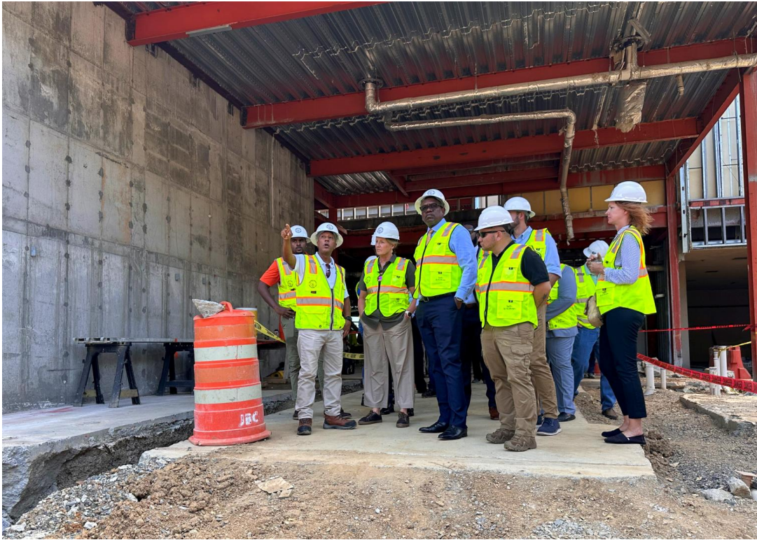
On July 30, Darryl A. Smalls, Executive Director of the Territorial Hospital Redevelopment Team provided FEMA Administrator Deanne Criswell, USVI Governor Albert Bryan Jr., and FEMA Region 2 Regional Administrator, David Warrington an overview of the restoration work happening at the Charlotte Kimelman Cancer Institute on St. Thomas. (Photo by FEMA/Deanne Swain)
