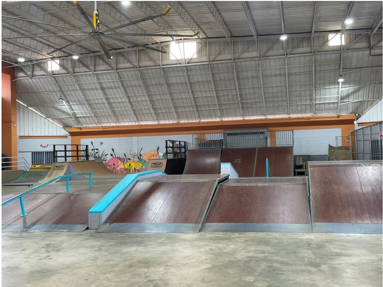
Rincón, Puerto Rico (December 13, 2023) – FEMA allocated over $812,000 to repair parts of the spectator area, the wooden ramp and the air conditioning system of the Rincón Skatepark. Photo FEMA/Zorymar Quiñones
