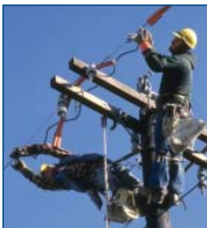
Power restoration is often the essential first step toward recovery after a disaster. FEMA works with its partners to restore public infrastructure damaged or destroyed by disaster.
