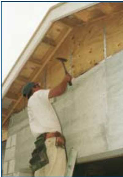
Structural reinforcements, like the hurricane straps being installed here, can reduce property damage from hazards such as hurricanes and earthquakes.
