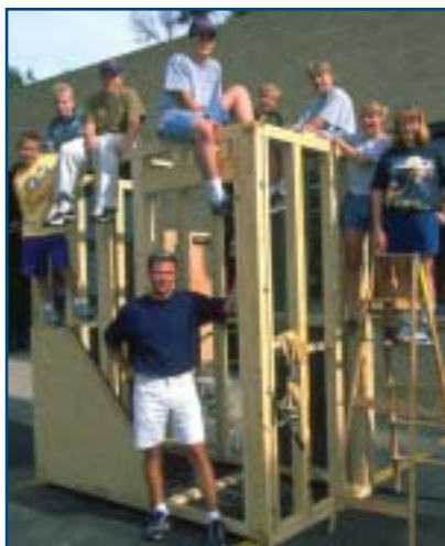
In Fort Morgan, Colorado, students build a safe room—a reinforced space within a home or other structure—to provide life-saving shelter during a tornado.
