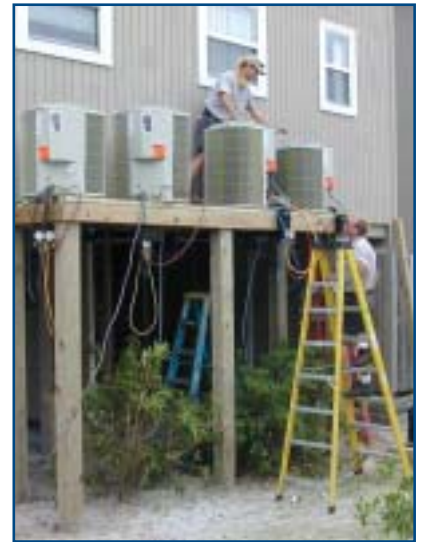
These workmen are installing new air conditioning units on a raised platform to replace the original units, which were washed away by flood waters. Good risk management decisions made before disasters strike can help avoid property losses.
