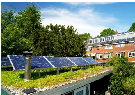
Combining solar panels with a green roof
