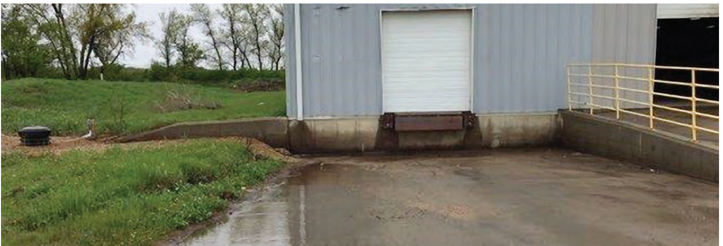
After installation of the winged culvert, which was successful in diverting water away from the loading dock.
