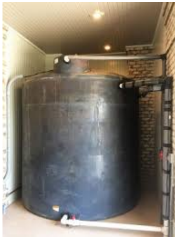
Figure 41. Example of a Covered Cistern in a Basement
